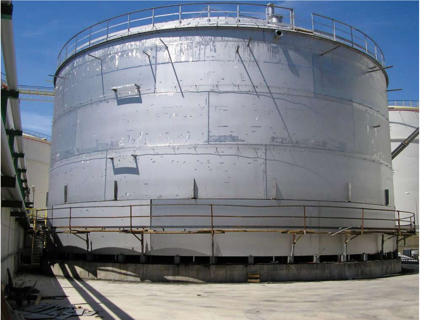
Figure 4: A pickled, duplex 2304 storage tank
