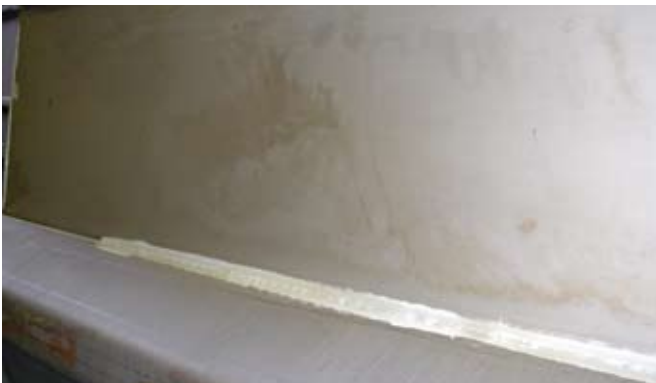
Figure 19: Dried-on pickling chemicals
