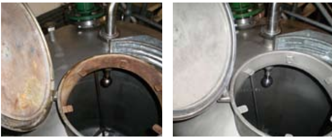
Figure 12: Surface rust – before and after removal using Avesta Cleaner 401.
